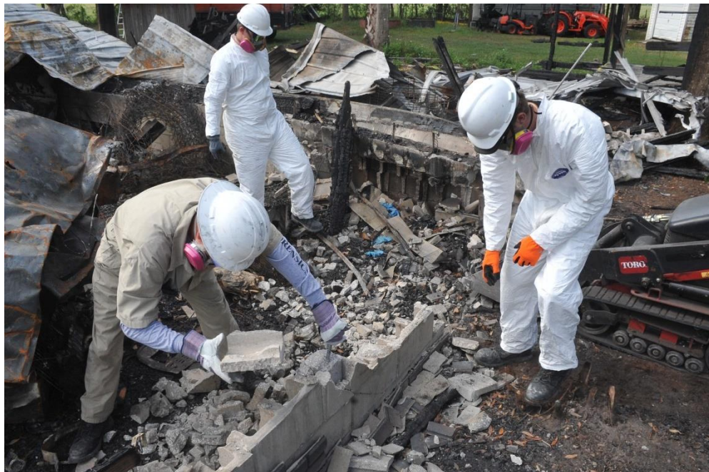
Figure 4 Private fire investigation team working in the post-fire environment. Credit: Kevin Hays Fire Consulting, LLC.
