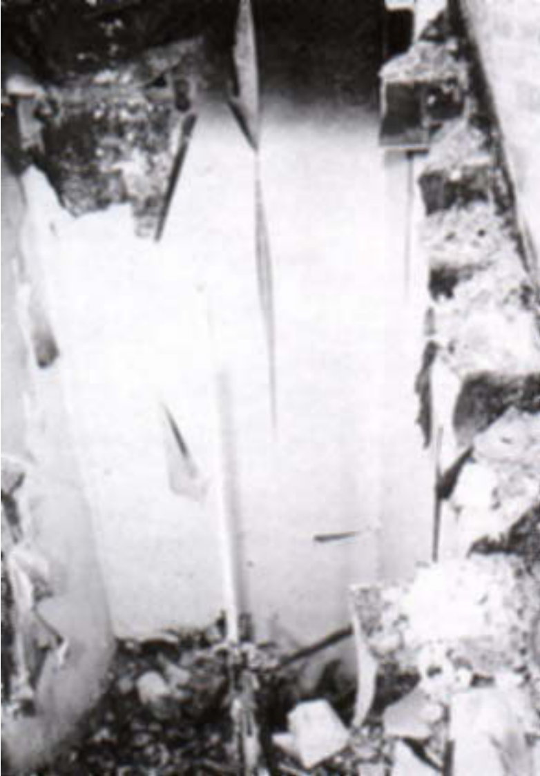
The stone stairs of this hotel in Bayswater, London, failed suddenly many hours after the fire was extinguished. A fire investigator was standing on the upper landing and fell, but fortunately suffered only minor fractures
