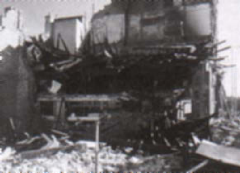
This large country house was gutted by fire, leaving the external walls unsupported...
