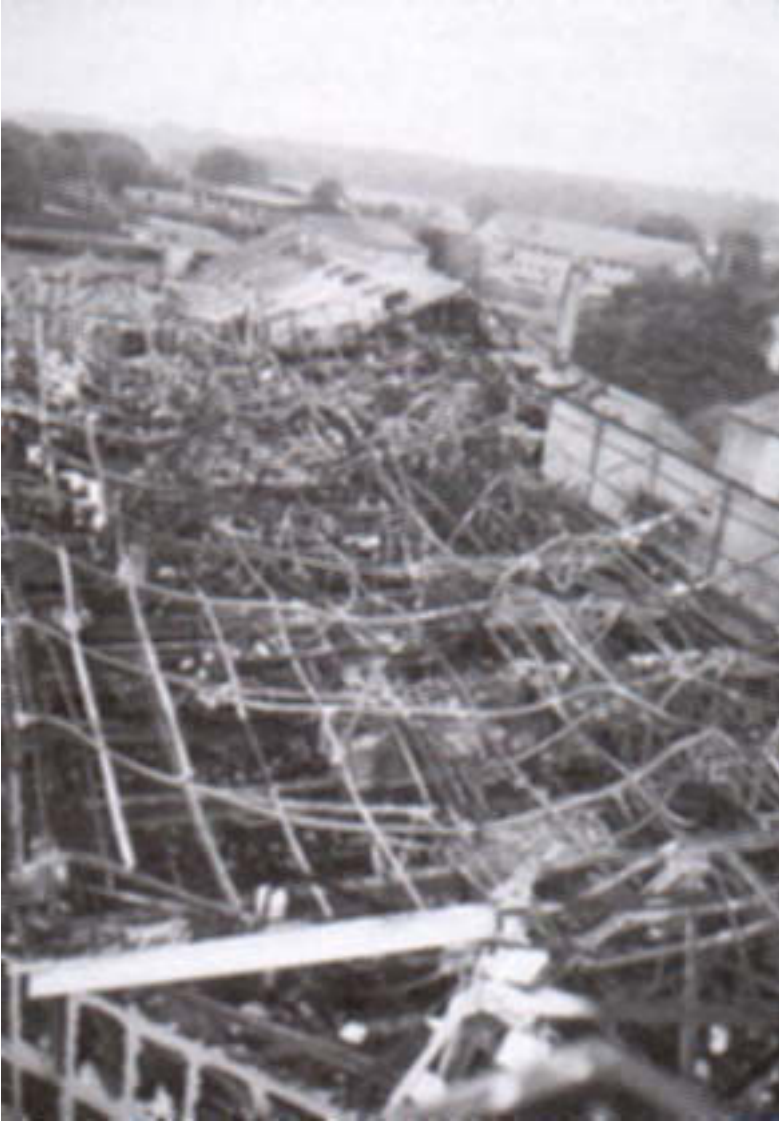
A large warehouse housed a printing works with heavy presses on the upper floor. Fire caused the steel roof structure to fail under its design load and caused deformation of the steel floor supports, allowing the machinery to hang into the area beneath.
